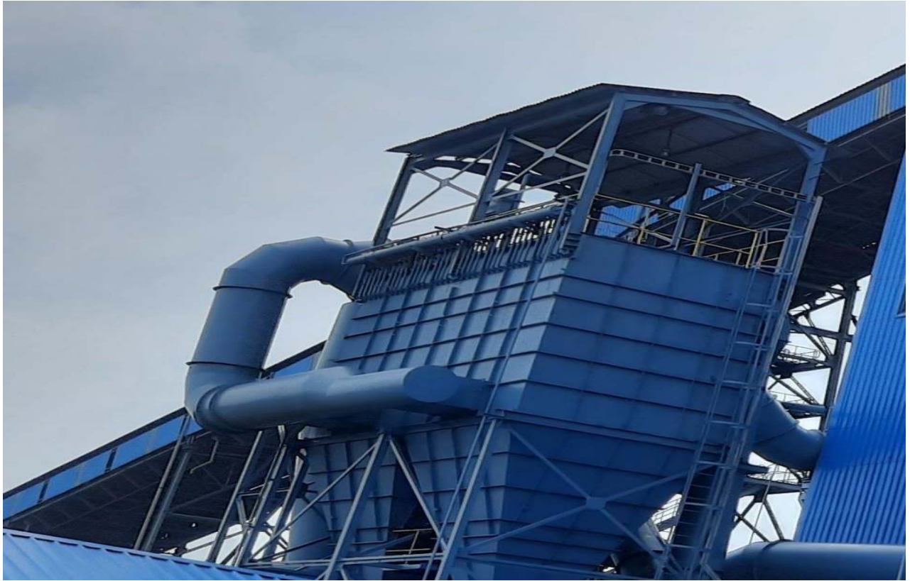
DUST EXTRACTION SYSTEM AT TRANSFER POINTS
